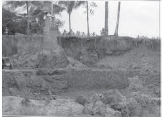
Damage to bank, infrastructure and change of river course
